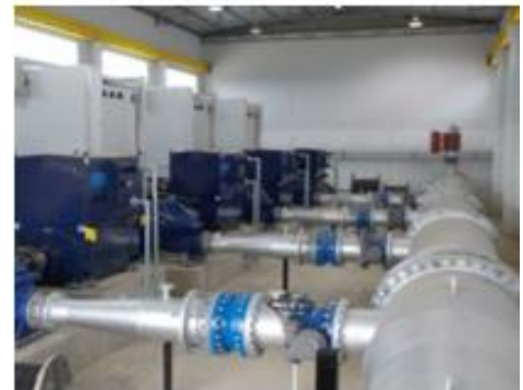
Fig. 3. Irrigation pump facility
